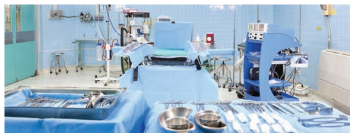
Figure 3. Modular clean room
