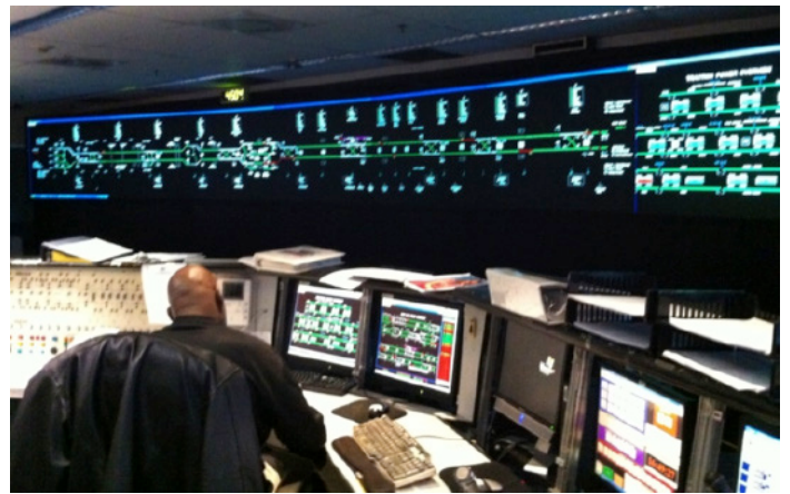
Figure 3. The metro subway control room inside the Maryland Transit Administration (MTA) Control center (4)
